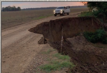
Wash out on Buckhorn Road
